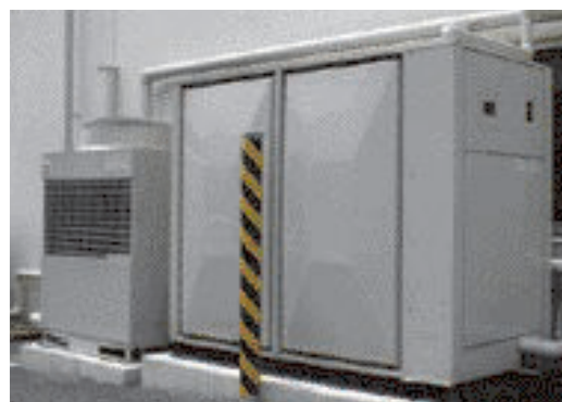
Regeneration tank (right) and outdoor unit containing a compressor (left)
