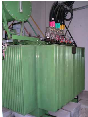
Municipal power (receiving) transformer
