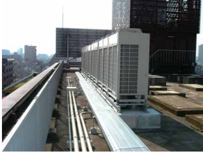
Outdoor units installed on the roof
