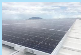
SMK Electronics (Phils.) Corporation Installation of Photovoltaic Power Generation Facilities
