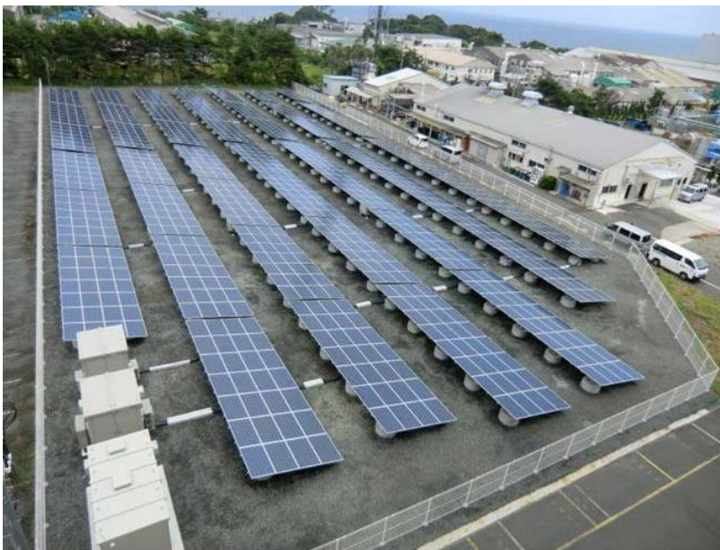
SMK CORPORATION Photovoltaic Power Plant Photo of Exterior
